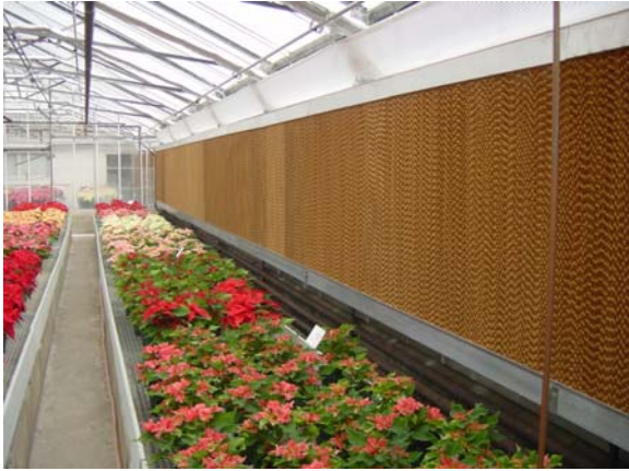
Figure 20. Evaporative cooling pad installed along the inside of the ventilation inlet opening. Photo courtesy of A.J. Both, Rutgers University.
