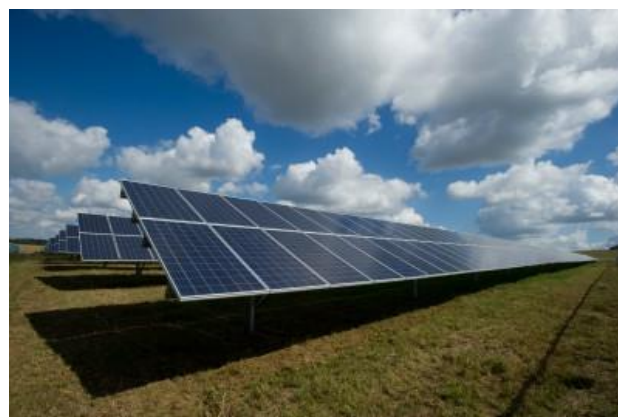
Utility grade solar projects are being sited throughout Michigan.
