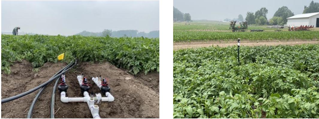
Figure 1. Installed Irrigation system, controlled by solenoid valves (Left). Xcel-Wobblers sprinklers by Senninger were used in this study (Right).
