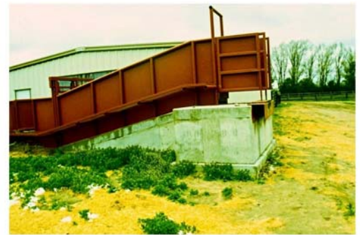
Cattle loading ramp with solid sides and a level dock
