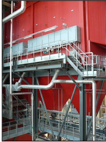
Large CHP plant boiler.
