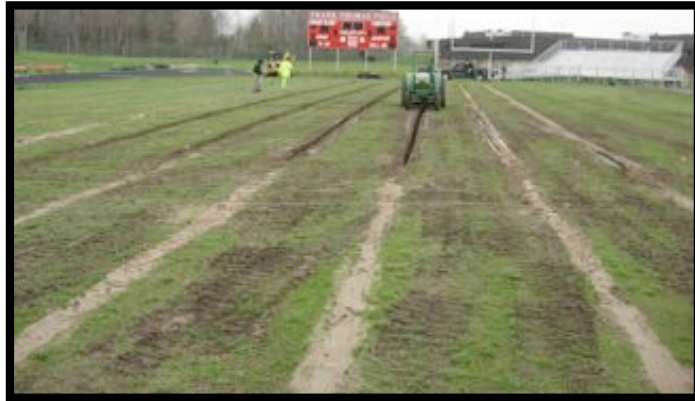
Image 1: Cutting drain lines, installing drain tiles, and backfilling lines with a sand-based root zone material, Grand Blanc High School, Grand Blanc, Mich., Water Management Inc., May 2007.
