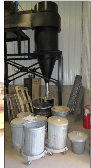
Ash is removed by hand. Cyclone separator behind.
