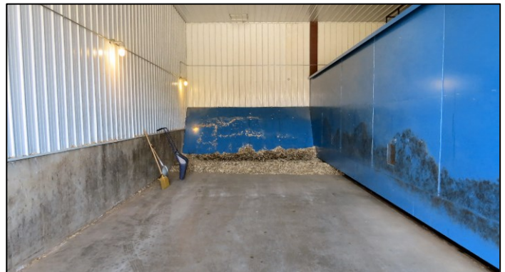
60-foot long chip storage bin, walking auger in back, under chips.
