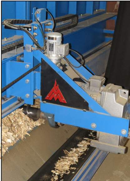
Walking auger feeds conveyor to the combustion chamber and boiler.
