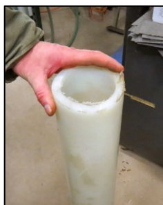
Piping used in heat distribution system, without insulation jacket.
